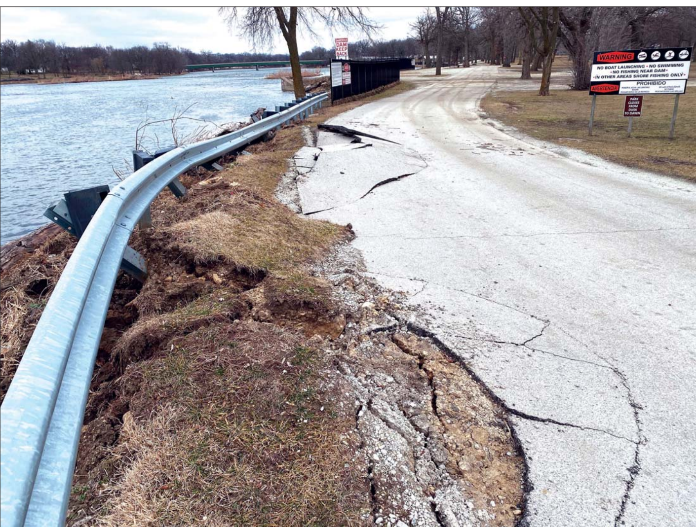
THE ROADWAY in the South Island park near the mill race bridge awaits repair after the guard rail and pavement were lifted during recent ice jams and flooding.
