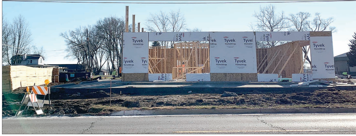
A DOMINO'S PIZZA restaurant is taking shape on the southwest corner of Division and School streets in the village of Diamond. Missouri-based MBR Management Corporation—conducting business locally as Domino's Diamond—is constructing a two-tenant structure at 2255 E. Division St. The pizza place will occupy one side of the building with a yet-to-be-named business on the other. The Domino's will have a pickup window, but no voice ordering box, according to information presented when the proposal went before the town board. Construction on the building began several weeks ago with an intended opening as soon as the end of the month. Mayor Terry Kernc has said that should the weather hold out, she has no doubt the business will be taking orders soon.
