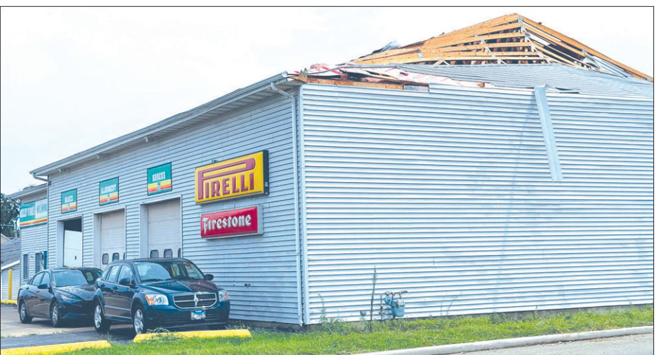
Photo by Eric Fisher A SECTION OF the rooftop at Tire Tracks, 507 W. Baltimore St, was lifted away by 100 mph wind or possible tornado on Tuesday around 11 a.m. Nearby buildings were mostly spared as debris from the powerful blast fell across two parking lots to the east.
